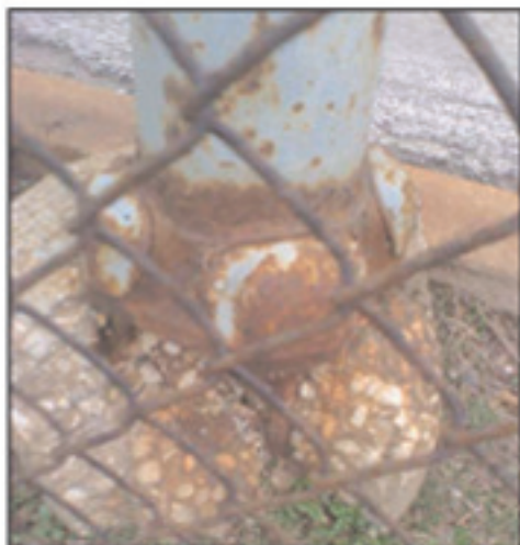
Example of light pole corrosion along Lake Shore Drive
